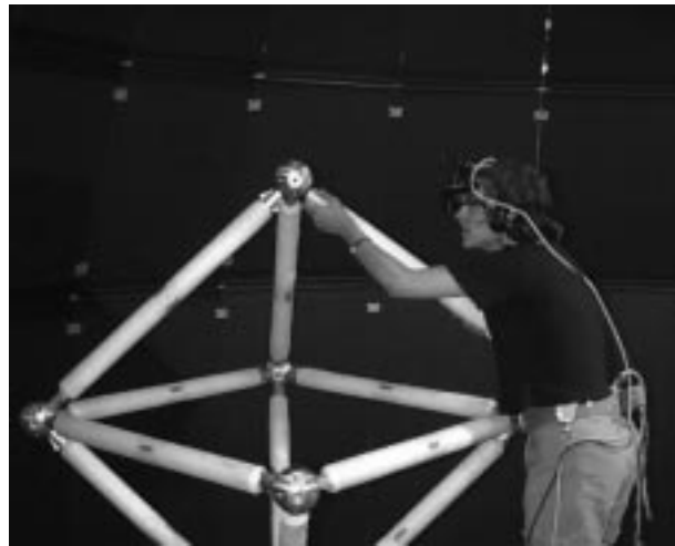
Figure 20.1 Prototype construction assistance system. The user wears a see-through head-worn display and a tool belt that serves as a holster for a hand-held barcode reader. Here, the user is following instructions to install a strut.
